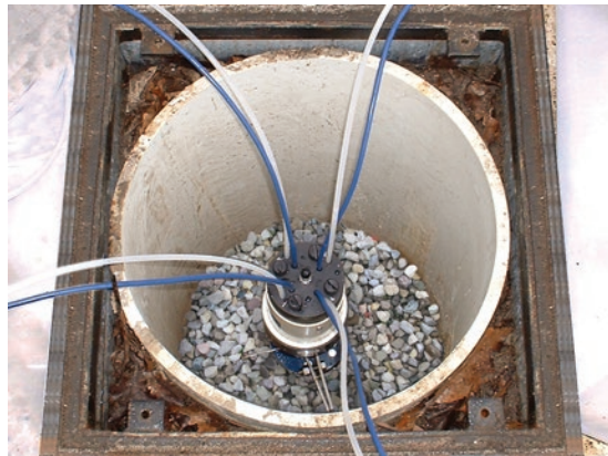
Figure 9-1 Tubing Organized Around the Wellhead
