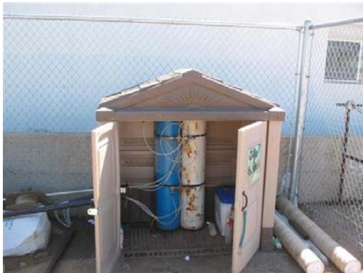
Photo 8: View of the shed housing the medical oxygen and the manifold system. Photo identifies the oxygen supply exiting the left side of the shed.
