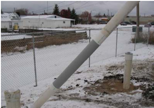
Photo 3: Photo of the Waterloo Emitter™ Monitor Well. Note the 2' section of solid PVC with a bottom cap to be used as a sump if needed.
