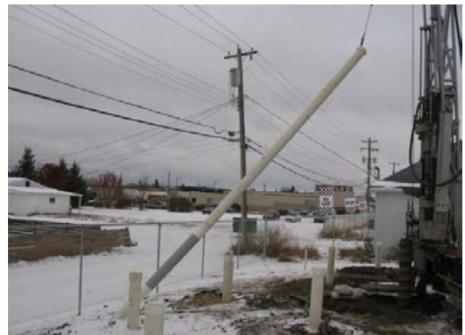
Photo 4: Installation of the Waterloo Emitter™ Well. Due to the weight of the PVC casing a hoist plug was utilized to install the monitor well safely.
