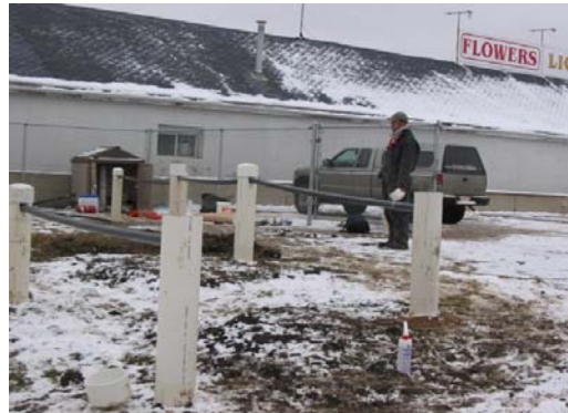
Photo 9: View of the above ground the Waterloo Emitter™ Monitor Wells. Each Emitter has its own dedicated LDPE line from the oxygen source. The LDPE line is enclosed in the ABS piping.
