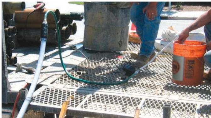
1" diameter Grout Line connected to Grout Adaptor, attached to bottom of CMT.
